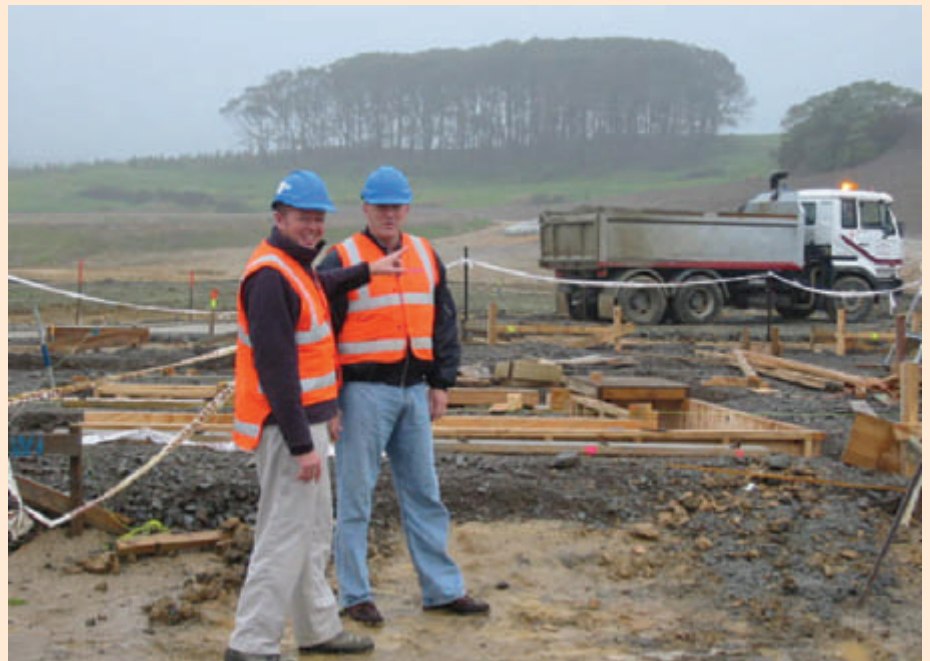
Construction Manager Duncan Kenderdine (left) shows Site Manager Mike Hughes some of the foundations being laid for the 350-bed Northland Region Corrections Facility.
